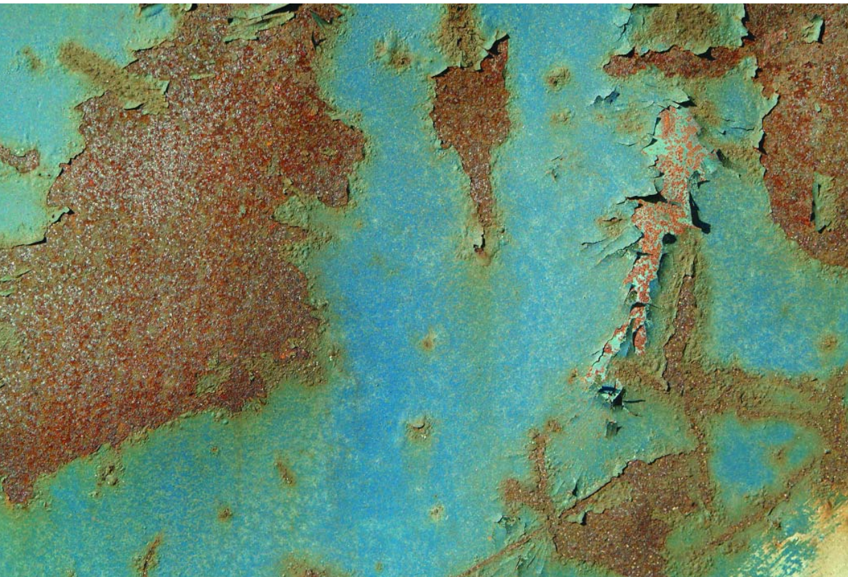
Fig. 1: Improper application and incorrect choice of coating material can have catastrophic consequences.
